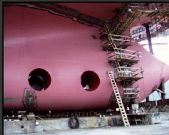
Scaffolding erected to test a weld line on the hull of a ship
