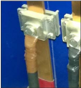
Fig. 3. An example of the type of bus bar tap-off clamp connection under observation.
